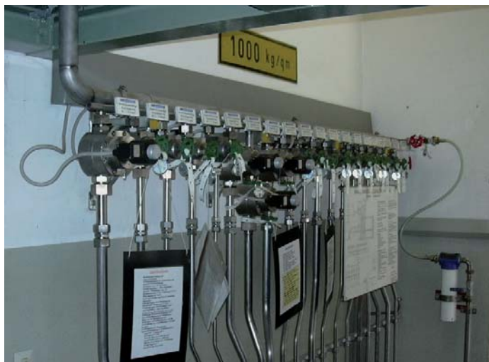
Fig. 4: Valve station at Bayer's Uerdingen (Krefeld) plant (source: FOGTEC)
