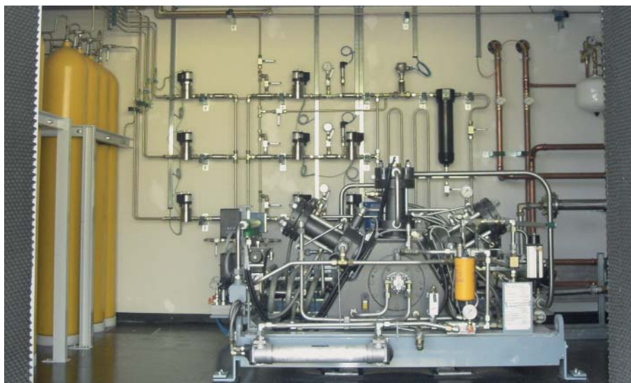
Fig. 6: Natural-gas filling-station facility featuring GSR high-pressure valves (source: RMG)
